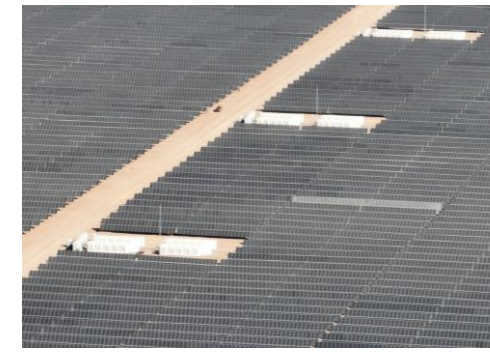
Andes Solar Ila & lib& IV | 398 MW Completed in 2020 and 2023
