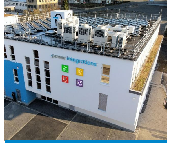
43 kW at Germany Facility
