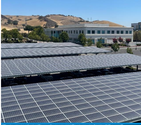
600 kW System at San José HQ Major Expansion in 2022-2023
