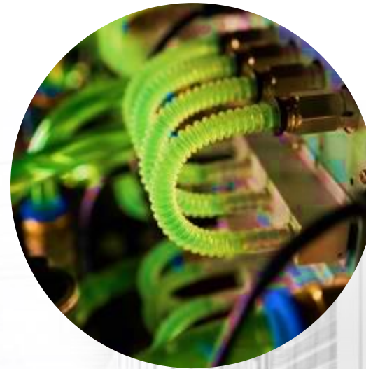
DATA CENTER INFRASTRUCTURE
