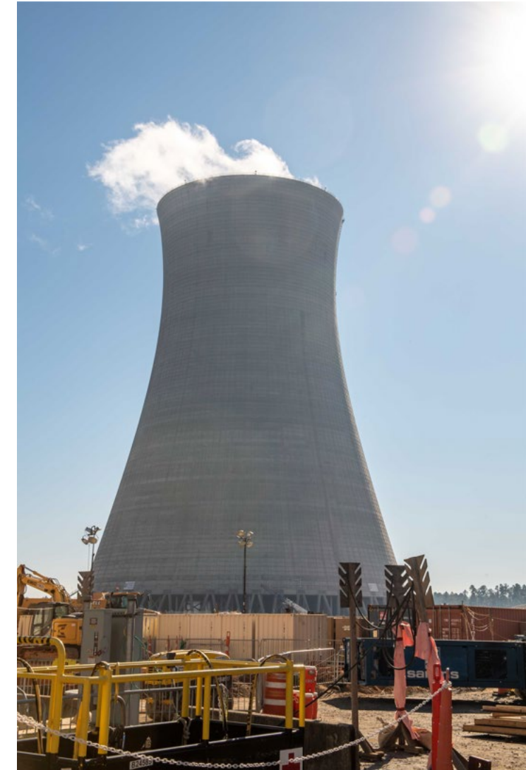
Unit 3 Cooling Tower during Hot Functional Testing
